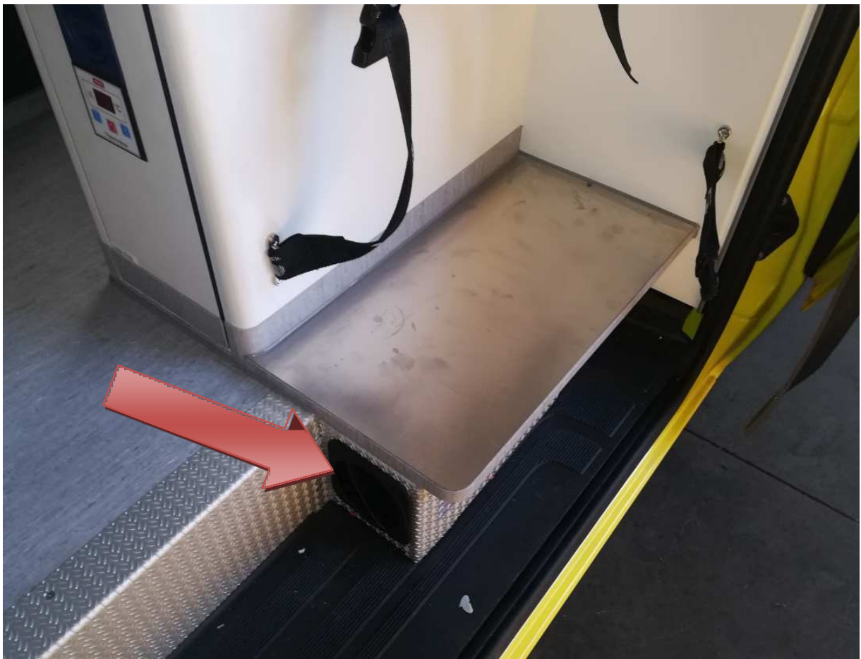
Fig. 20 Location of the warm air diffuser
