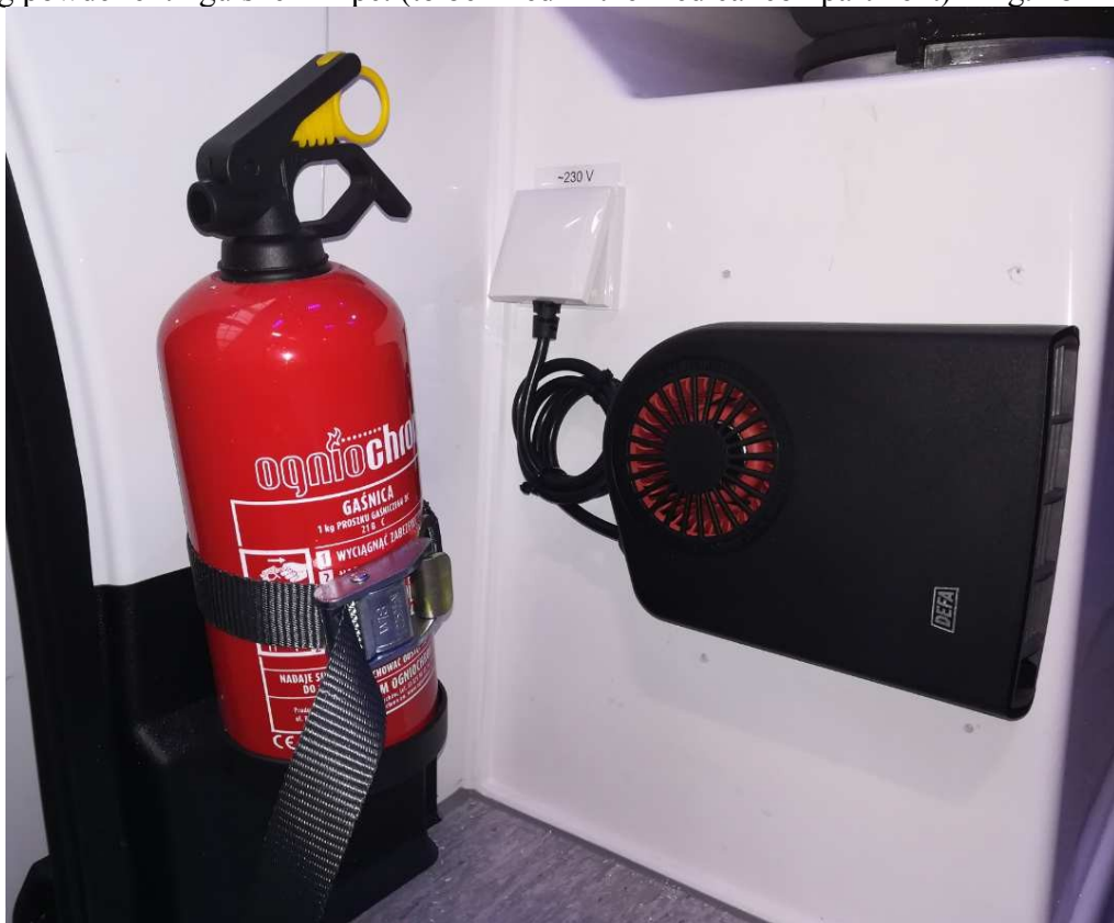
Fig. 48 Medical compartment fire extinguisher
