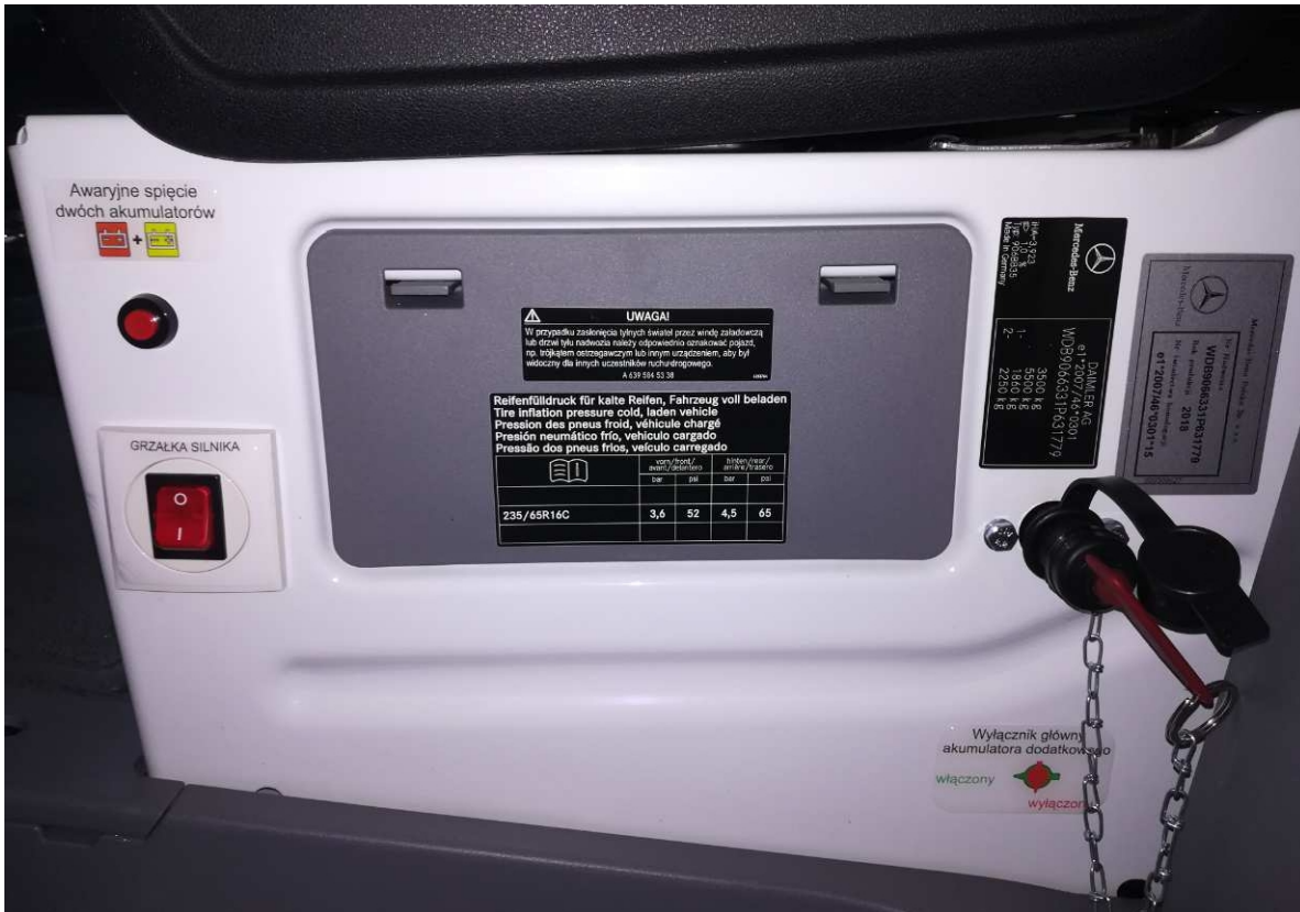
Fig. 13. Auxiliary battery switch
