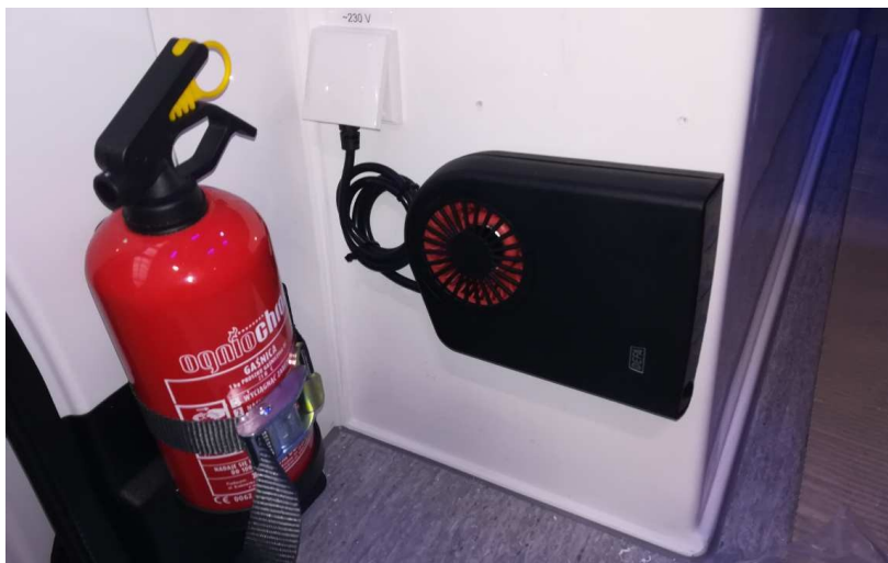
Fig. 25. Location of stationary 230V mains-powered medical compartment heater (DEFA 2100 W)
