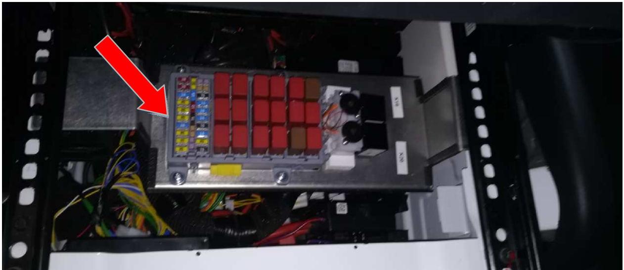
Fig. 67 Location of fuses under the driver's seat.
