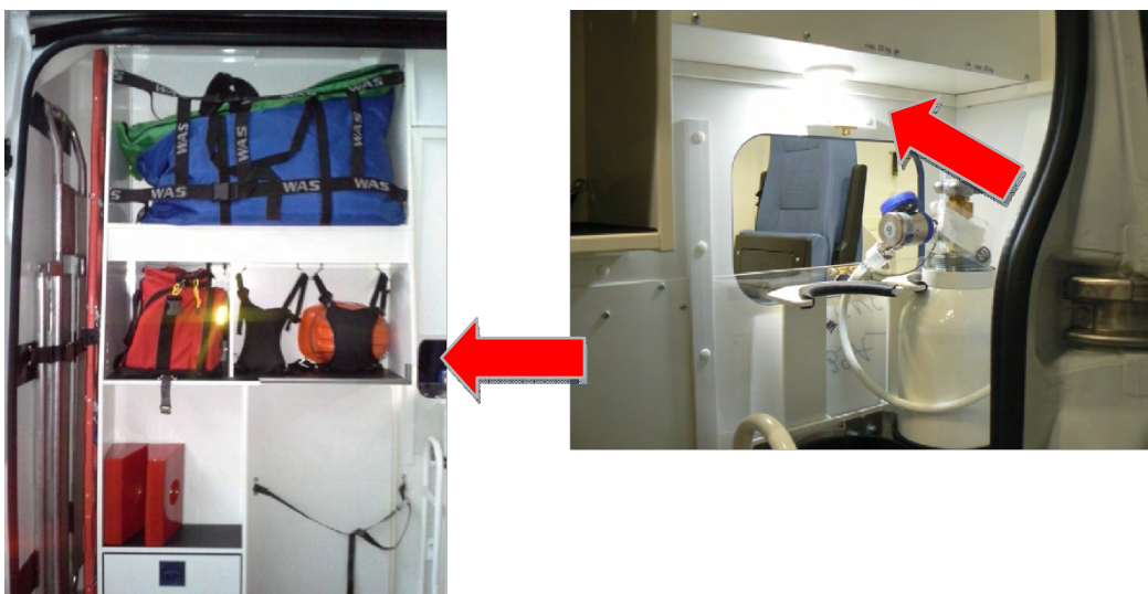
Fig. 34. LED lighting of the technical compartment
